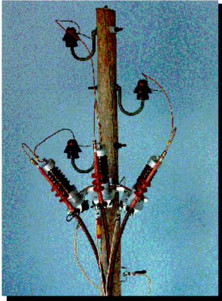
Porcelain housed surge arresters of type MWB protecting cable end terminals
